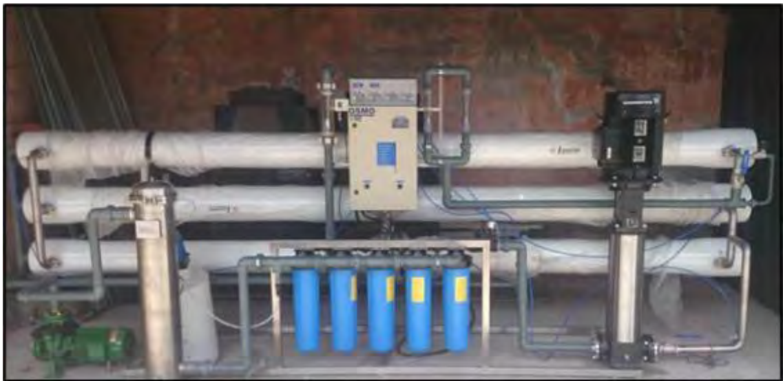
Figure 145: Reverse osmosis water treatment plant.
