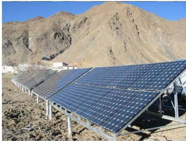
Fig. 25 Solar energy photovoltaic power generation system in the Qinghai-Tibet Plateau
